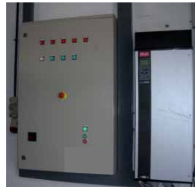
Example: wall mounted panel
