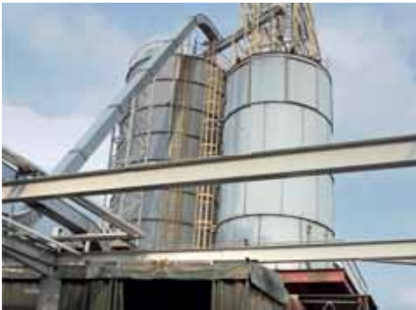
Chain conveyer from filter to silo
