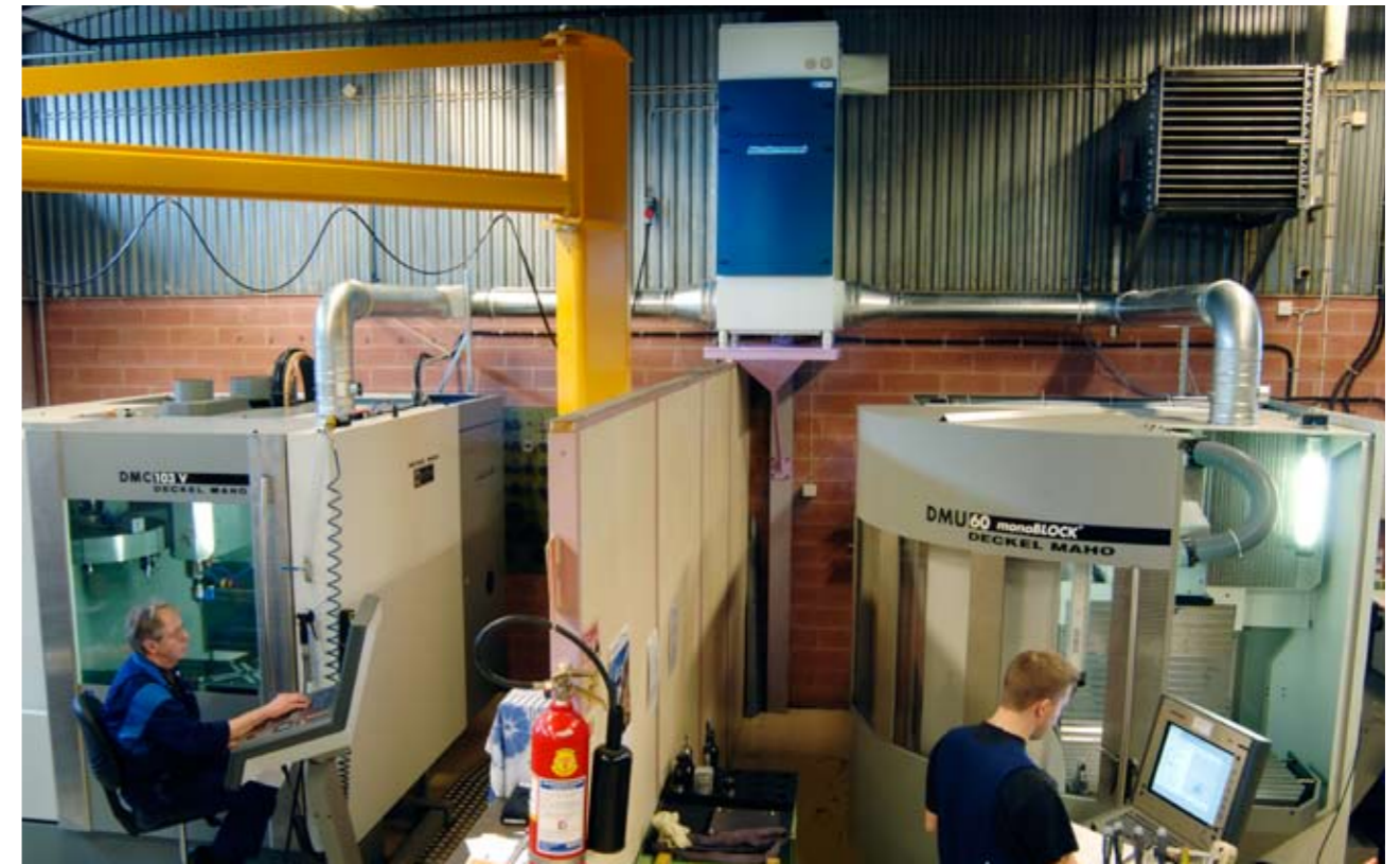
By removing oil mist at source it will be prevented from settling on sensitive electronics or other surfaces in the workshop, disrupting production and creating hazards.
